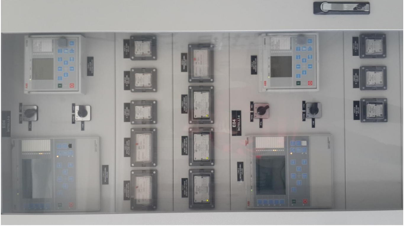
Ambarlı 154kV Relay Panel
