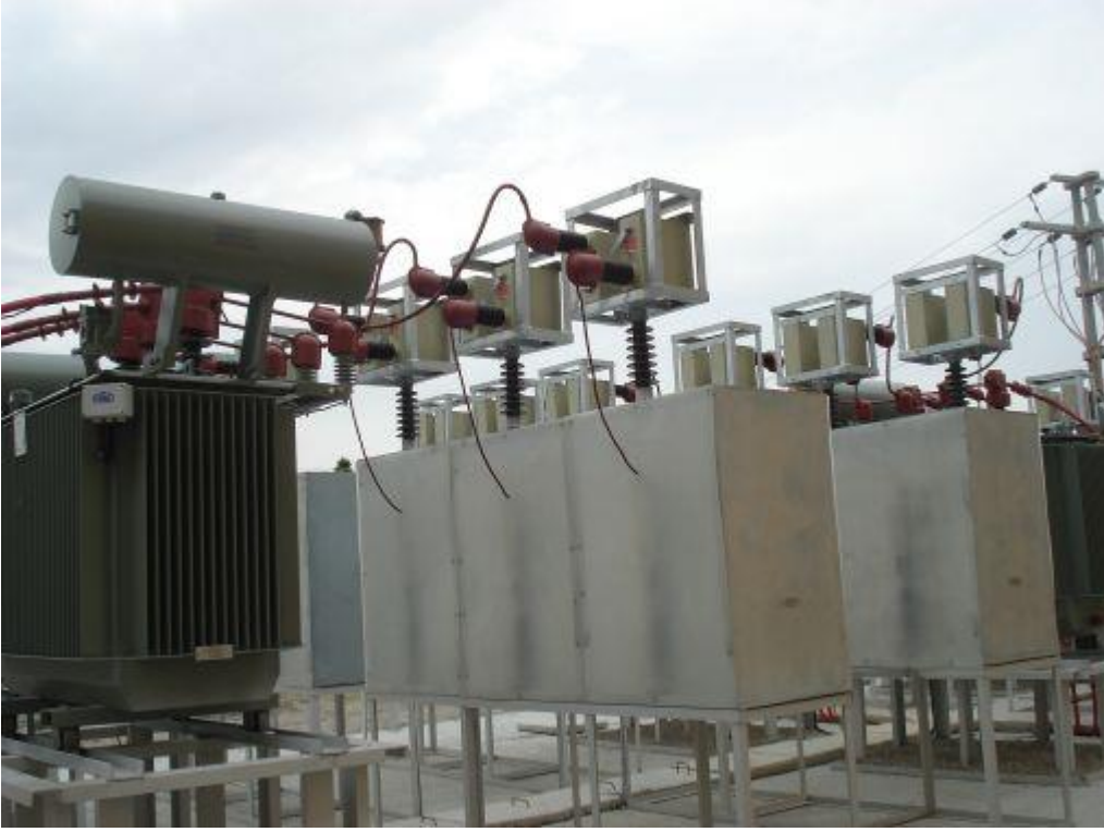
Turkey's first MV automated shunt reactor systems- 2010
