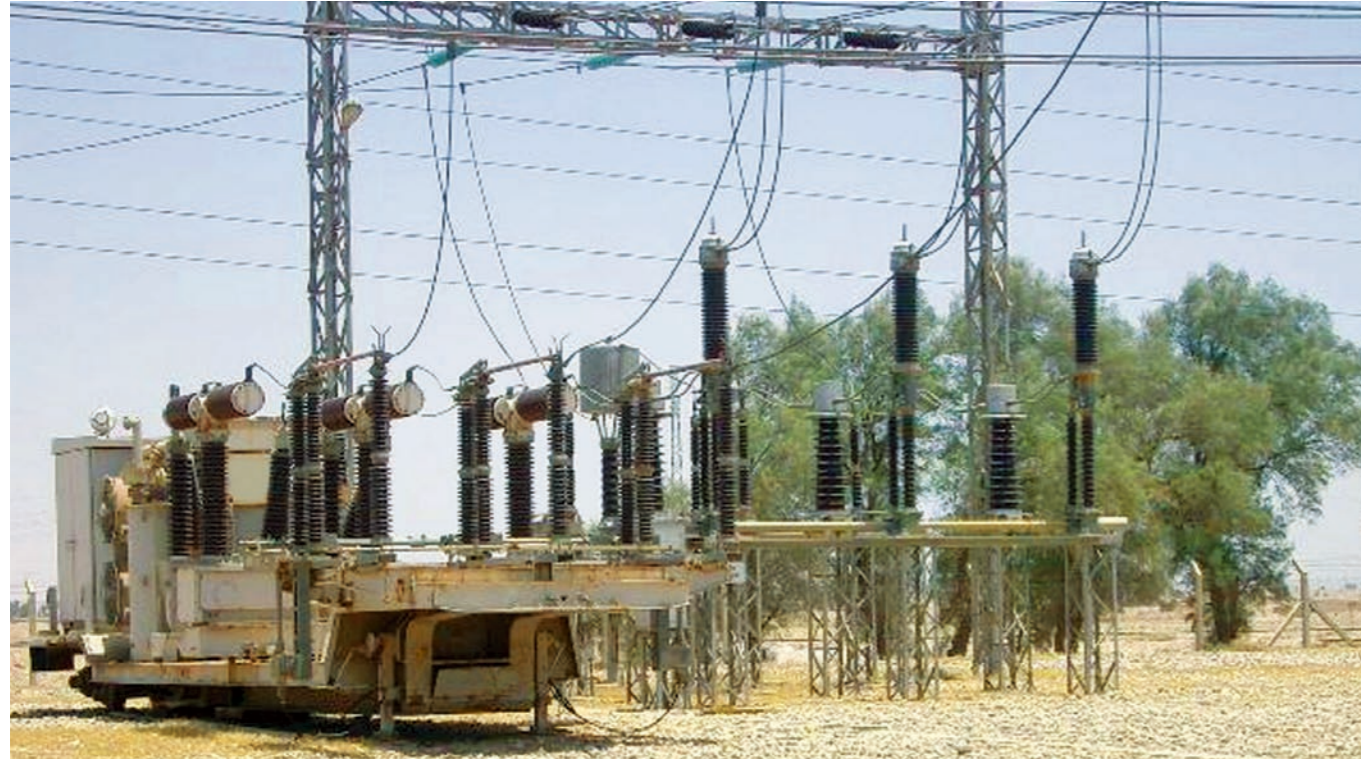
132/11.5kV Compact 10 MVA Mobile Substation (All in one trailer type)
